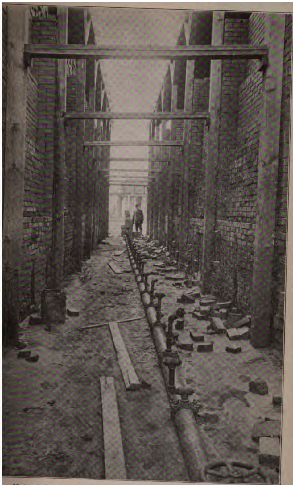
Natural Gas Line at Plant of Northwestern Brick Co., Wichita Falls, Wichita County.
